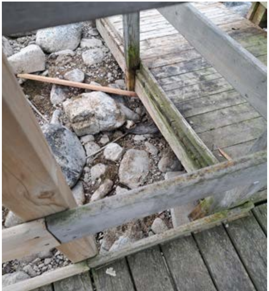
Dead Salmon trapped under decking
