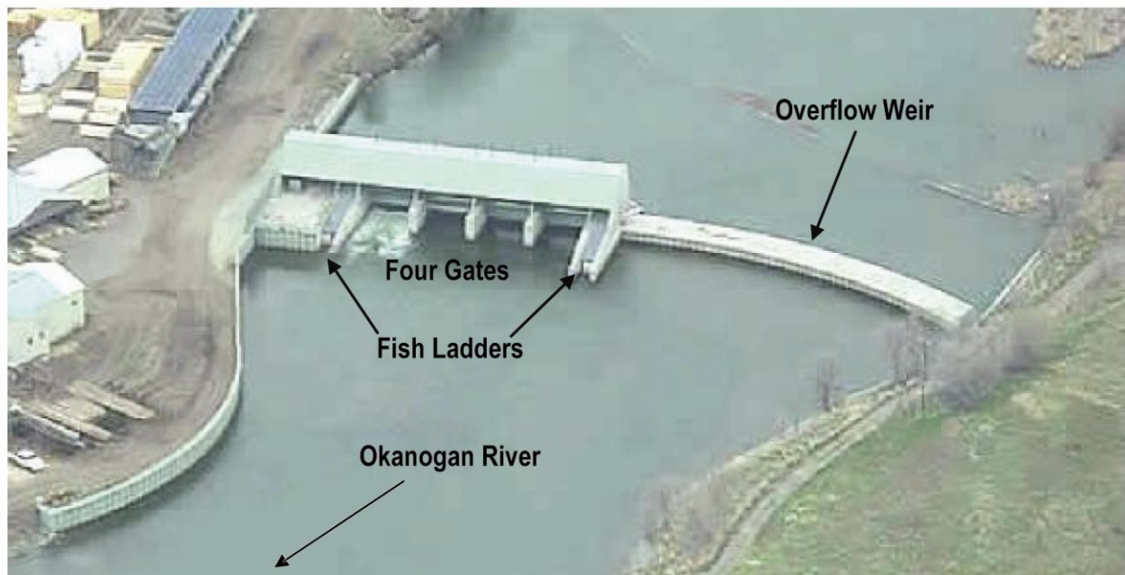
Figure 2. Aerial view of Zosel Dam showing the control structure and overflow weir. (After Summit Environmental Consultants, 2010a).
