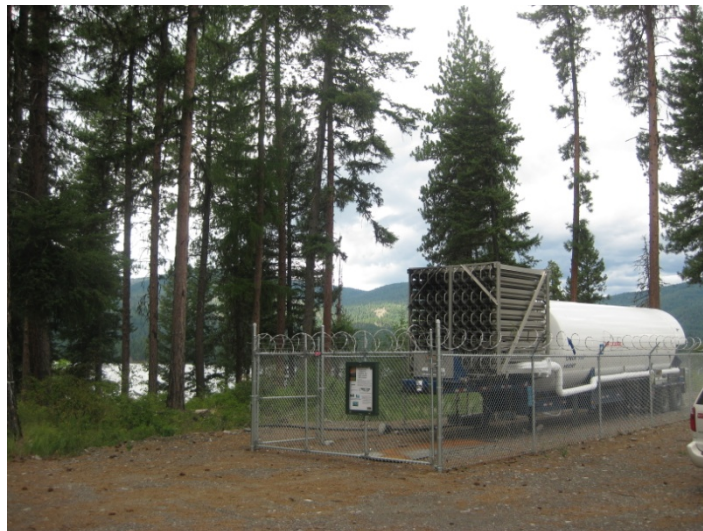
Figure 19. On-shore oxygenation facilities at Camanche Reservoir, CA (top) and Twin Lake, WA (bottom). Both systems include a liquid oxygen storage tank and an evaporator to convert the liquid to gaseous oxygen. The gas is then piped down into the bottom of the lake. The Camanche system uses a submerged contact chamber while the Twin Lakes system uses a line diffuser. See Beutel and Horne (1999) for a review of lake oxygenation technology and water quality improvements.
