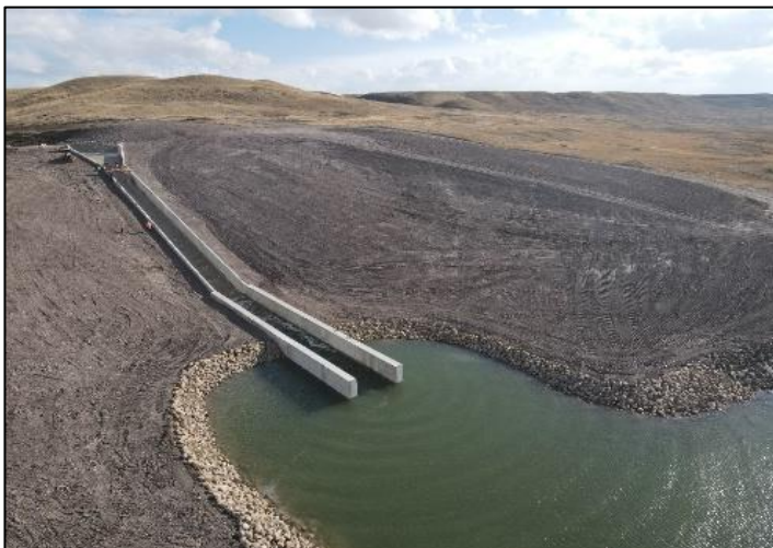
Reconstructed Drop Structure #5 on the St. Mary Canal, just before it joins the North Fork Milk River, Amskapi Piikani territory, October 2020 (from Montana DNRC Factsheet )
