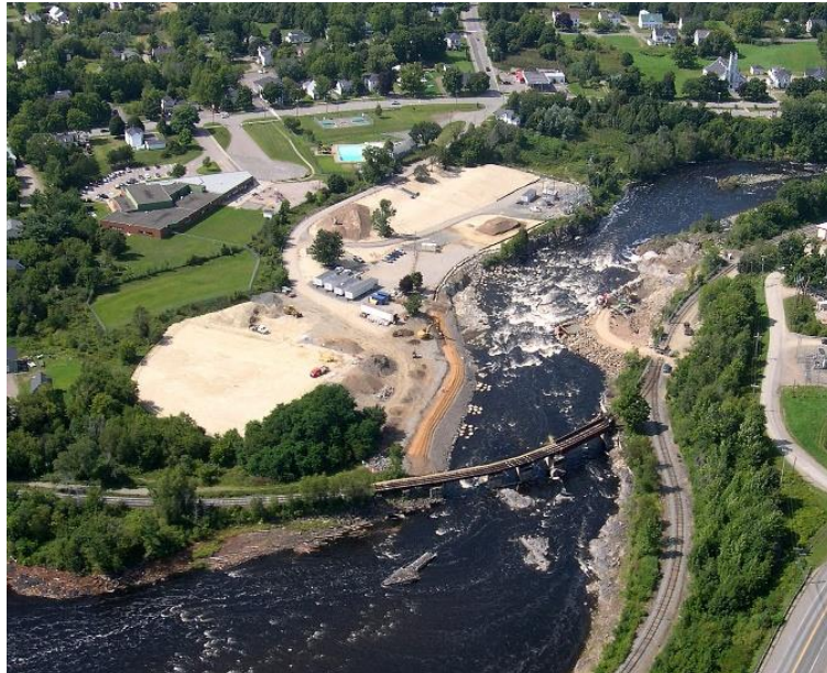
Figure 10 Milltown Generating Station (MGS) decommissioning and Salmon Falls restoration as of August 28, 2024. Photo credits: Ed Friedman from Point of View Helicopter Services.
