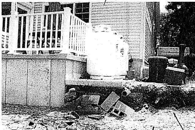
unprotected Erosion propane tanks
