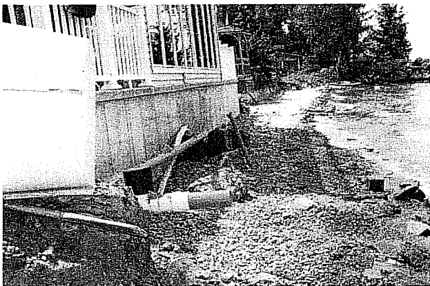
pipe destroyed March 2005
